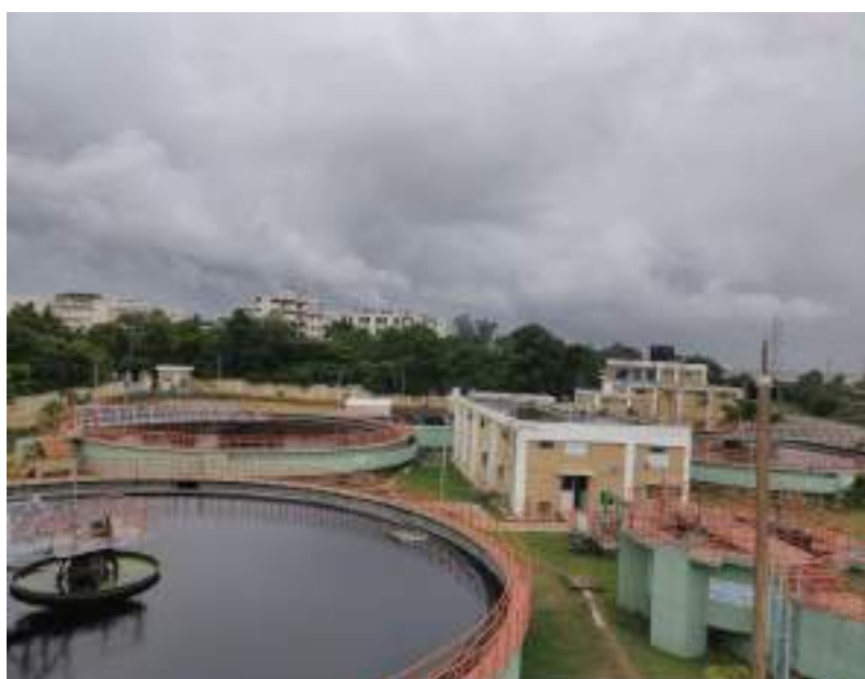
36 MLD STP at CDA-Bidanasi area of Cuttack
